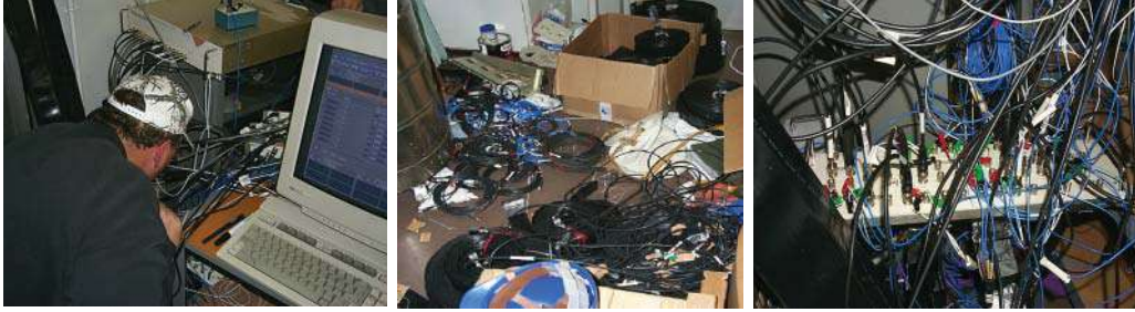
Figure 10.4 Test setup with a “rats nest” of cabling.
